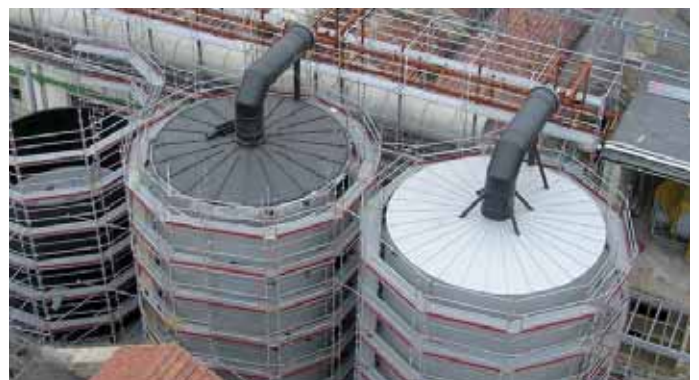
13 meter high silos was made of HDPE, Spain
